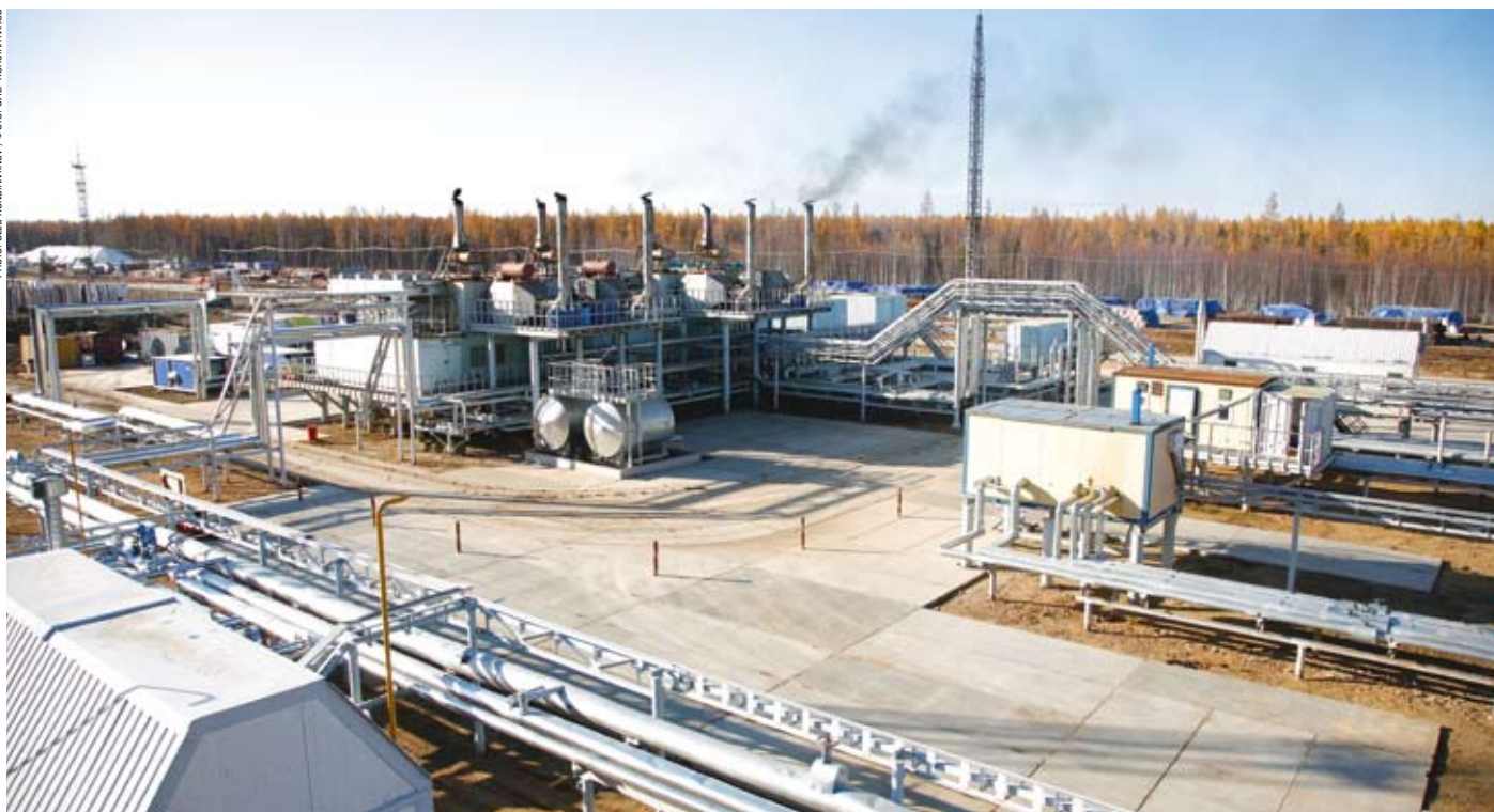
Phase One of the captive power complex fed with associated gas is already in operation in VC field. ▲
